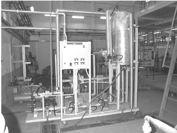
Fig. 3: PARS-EX pilot plant
