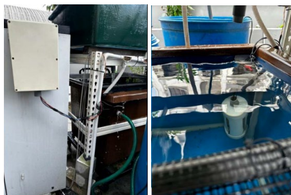
Figure 6. IoT Monitoring System installed at site
