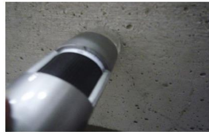
Fig. 6. Measuring crack width using Dino-lite digital microscope.
